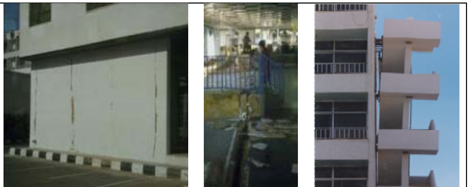
Figure 1: Pictures showing the minor damage and cracks due to the 1995 earthquake in Aqaba City.
